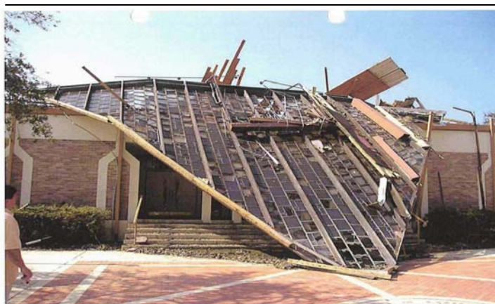
Our Lady of Lourdes Slidell, LA Wind and storm surge Hurricane Katrina
