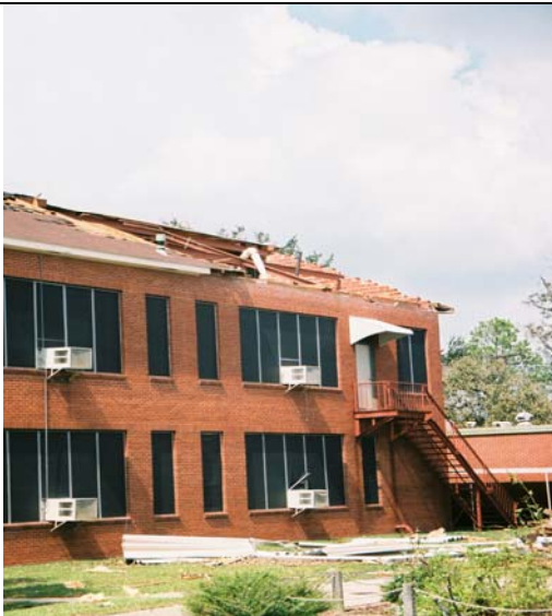
Immaculate Conception Groves, TX Wind damage Hurricane Rita
